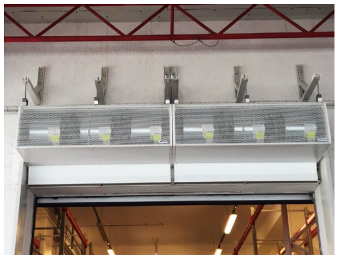
Fly KXL Installation in a dairy products factory
