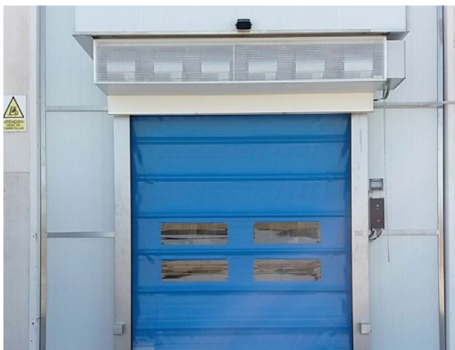
Fly KXL Outdoor installation in legume factory service door
