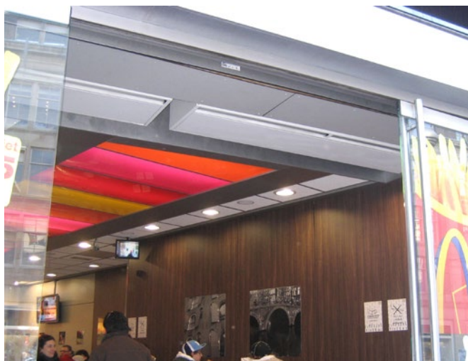
Fly K Multiple installation in a fast food restaurant
