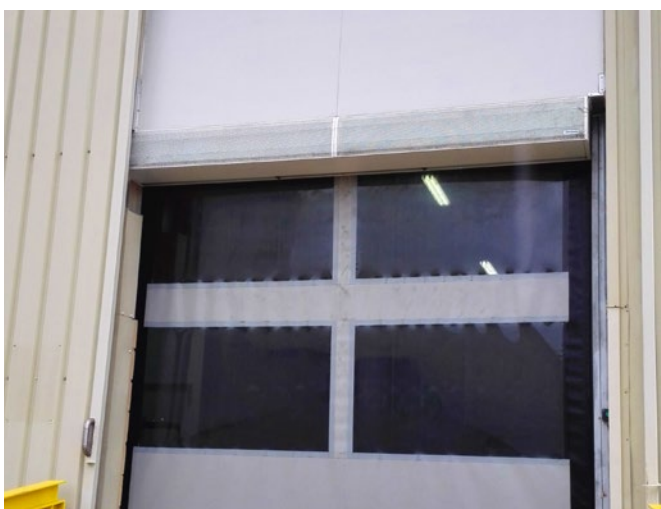
Fly KBB Multiple outdoor installation in a pharma factory doorway
