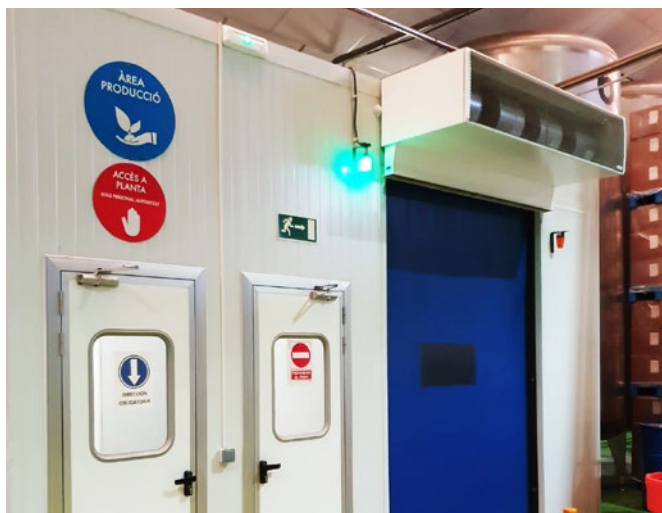
Fly KXL Installation in a honey production factory
