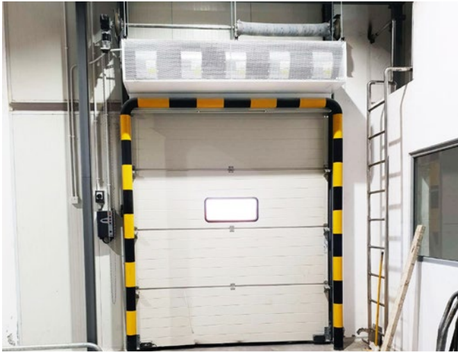
Fly KL Installation in a bakery factory service door
